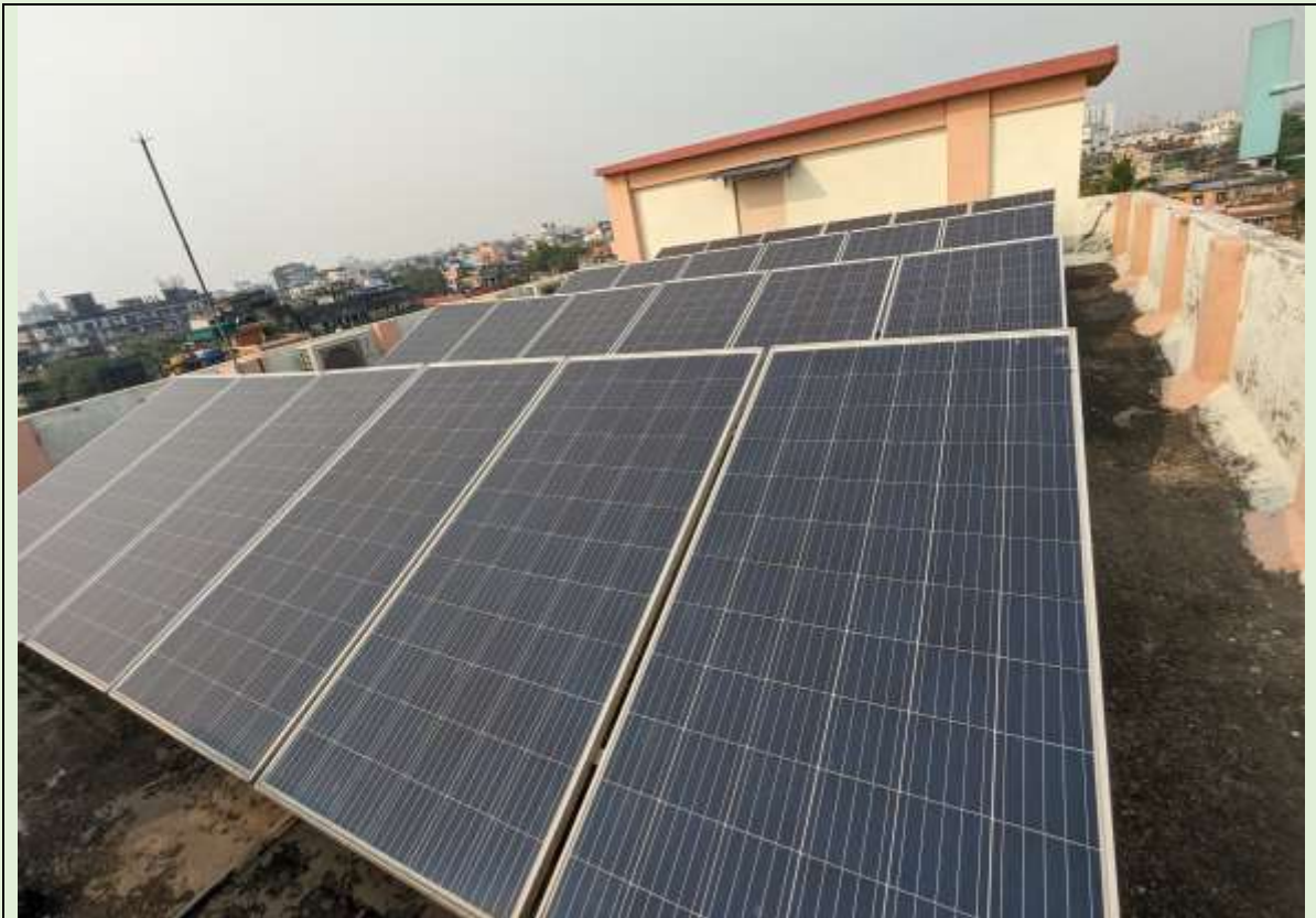
Installed Roof Top Solar Panel
