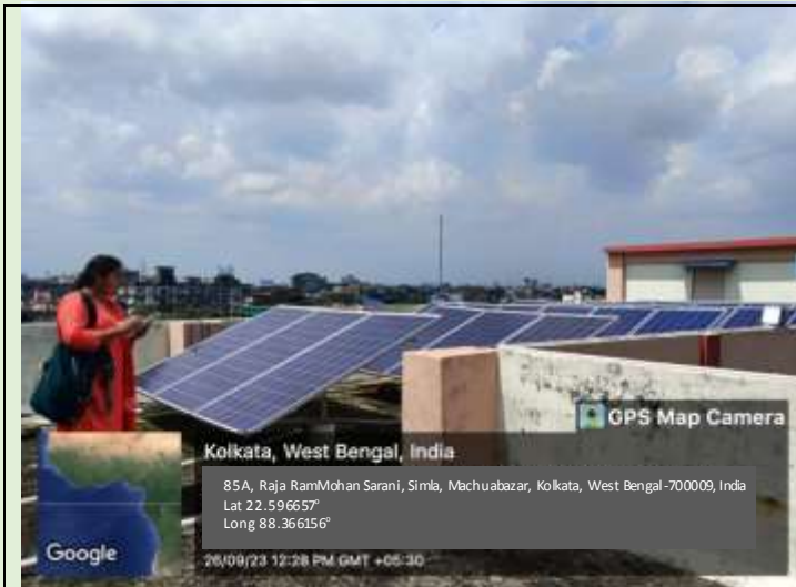
Installed Roof Top Solar Panel
