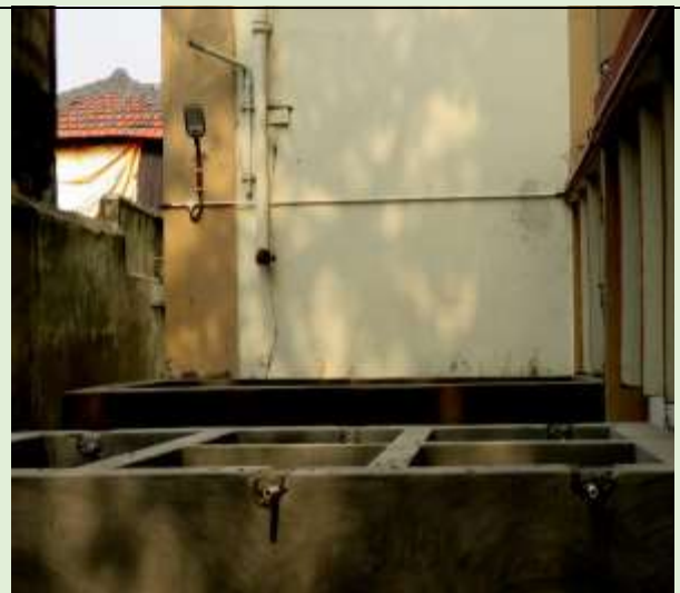
Modified Rain Water Harvesting System
